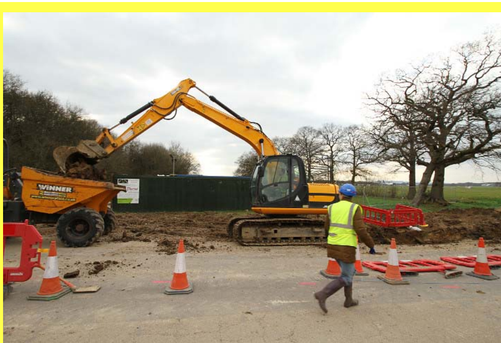
The Trust's newly-acquired 13ton JCB excavator is already being put to work near the new Compasses Bridge, digging the access road foundations (picture: Julian Morgan)
