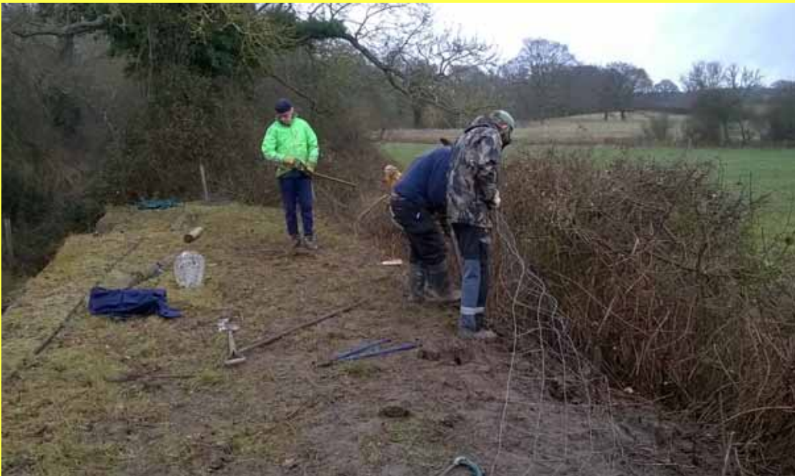
This page and next - three images of Monday Group hard at work clearing brambles and undertaking other tasks at Malham Lock on 19 February. (Pictures by Martin Burgess)
