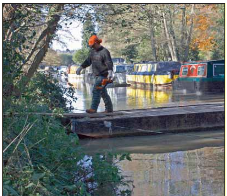
Because of access restrictions, initial clearance work at Gun's Mouth Island had to be carried out from a pontoon. (Janet Phillips)
