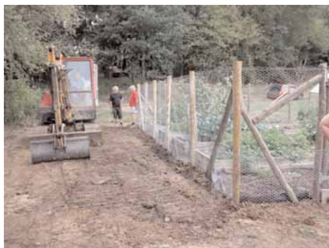
Summer camp 2010 - work included moving fences, glasshouses, horse troughs etc to provide access to Southland Lock (Allan Chambers)
